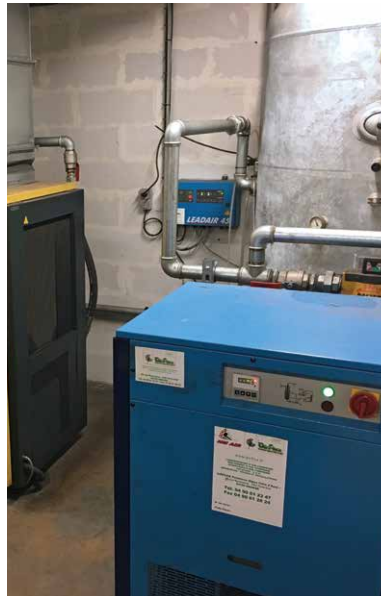
New compressed air system
