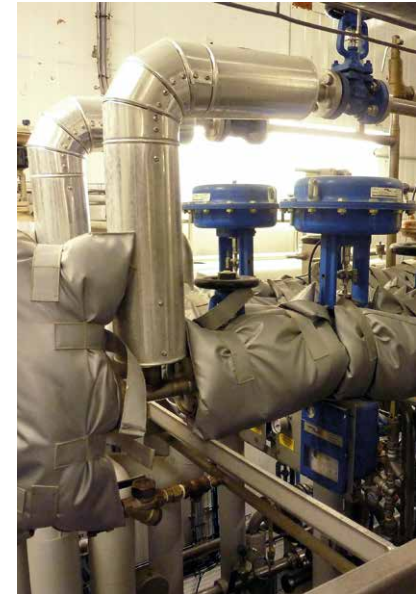
Steam valve insulation
